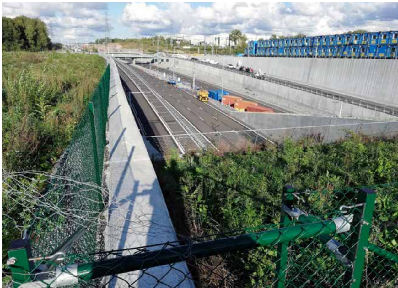
Figure 37. The bypass is laid in a tunnel not only where it crosses the green wedge of Järva but along most of its 25 kilometer long stretch. Photo: Richard Murray.
